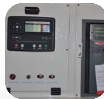
Control Panel & MCB
